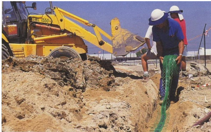
Marker tape being installed in the trench above the pipe (photograph courtesy of Iplex Pipelines)
