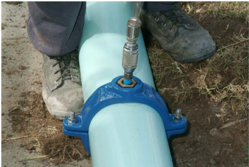
Coated Ductile Iron saddle, dry tapping using hole saw in a brace and bit to cut the hole.
